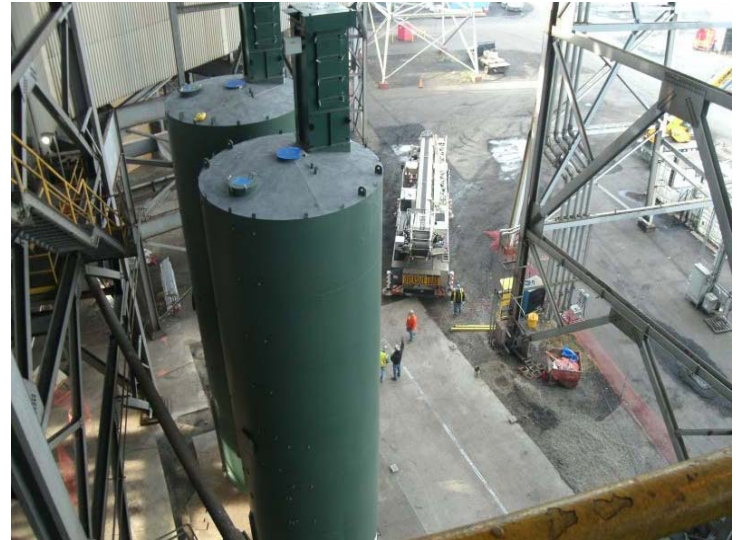
Example Sorbent Storage Silos
